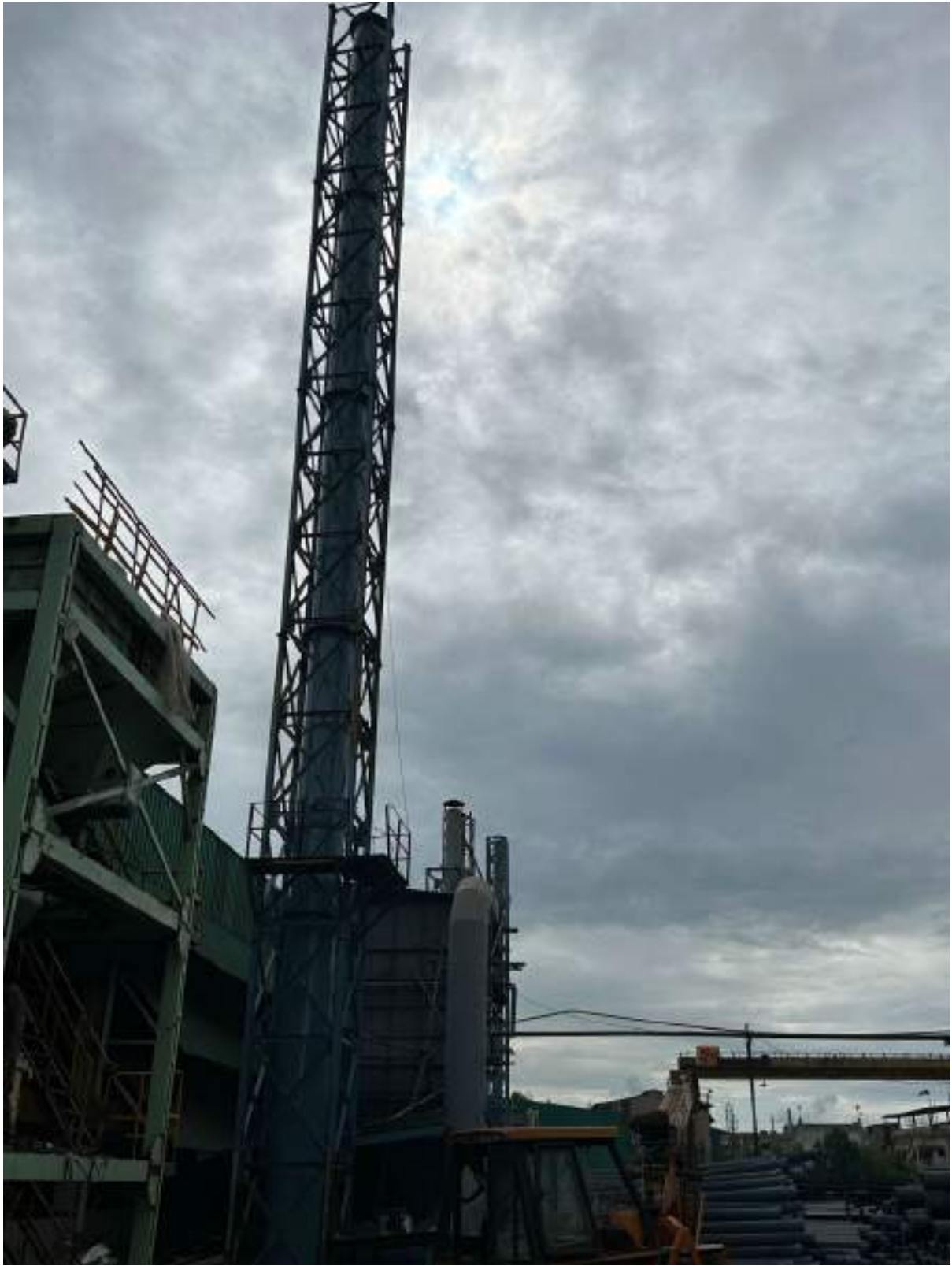
ZINC COATING CHIMNEY AND BAG FILTER
