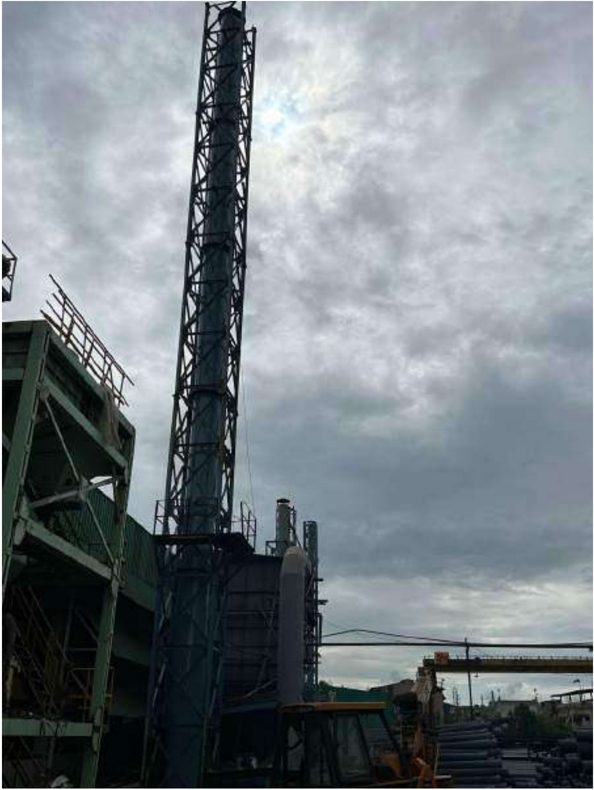
ZINC COATING CHIMNEY AND BAG FILTER
